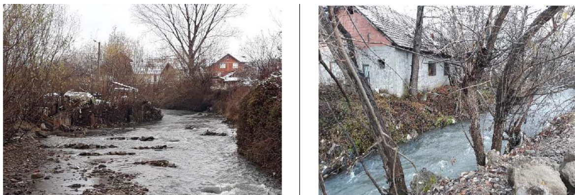
Figure 3: Narrowing of the watercourse by private facilities in the river bed
