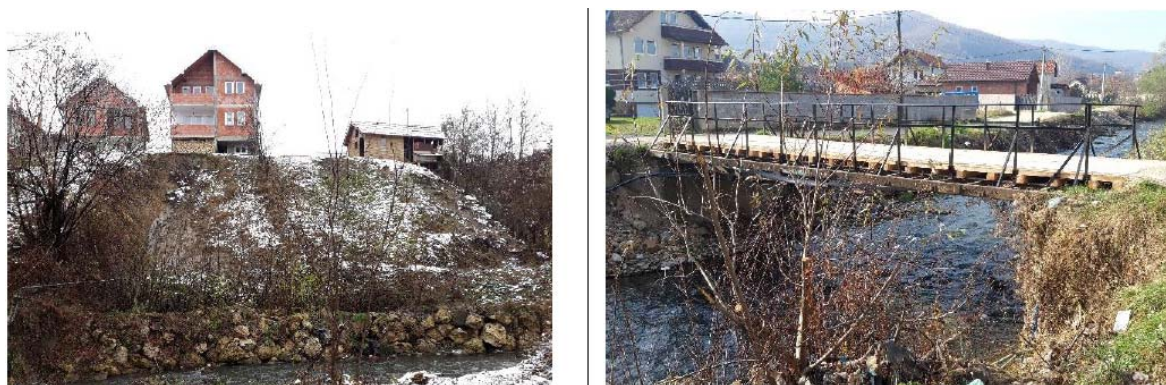
Figure 8: The instability of the river banks and the suspended bridge on Raska
